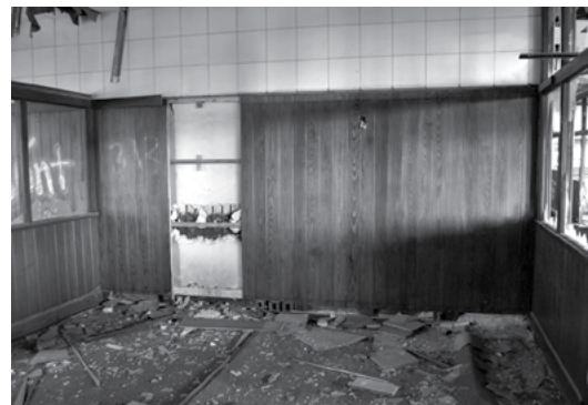
The Good. The Bad. And, the Ugly: Some of the offices had 8’ walls of paneling. Working in the old building held danger from the years of trespassing and abuse with broken glass everywhere.
