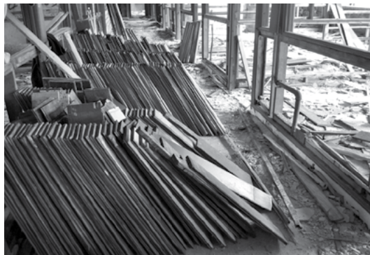
Stacked and Ready to Roll: As the contractors began to take the offices apart, they would have pile after pile of wood to carry downstairs and load into Ulrich Lumber trucks. The salvaged items were transported to a warehouse on the Packard Proving Grounds located in Shelby Township, Michigan.
