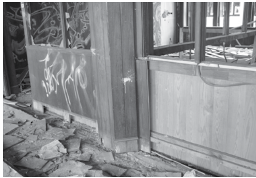
Beauty and the Beast: Another example of how beautiful the original wood is! On the left you can see an office wall as it was found... On the right you see the virgin wood after removing the outside wall. It was really exciting for the crew to see!
